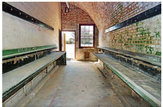
Ablutions casemate showing recent use as battery charging station for Connaught barracks. Photo Bob Clary
